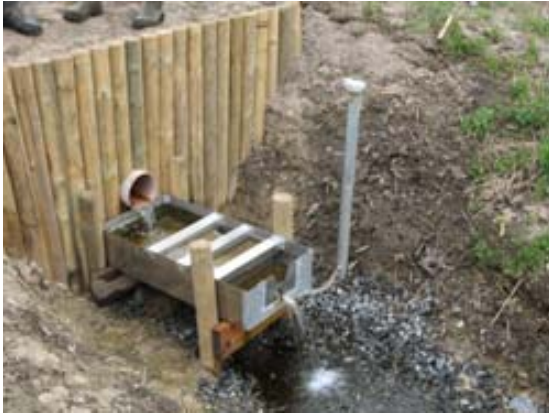
Main drain and gauging weir
